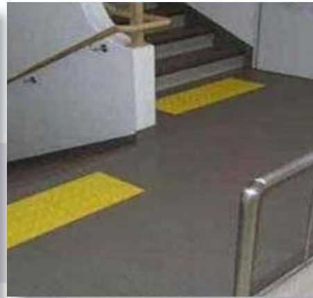
Figure 37 - Warning Blocks at Landings
