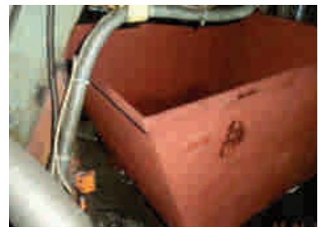
As shown below, Conveyor sensor provided
